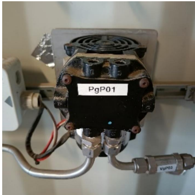
Figure 4: Syngas pump for solar gas intake.
