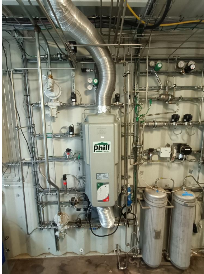
Figure 13: Gas intake and compression section.
