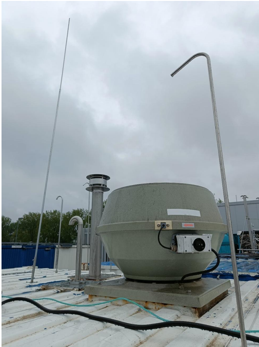
Figure 12: View of the roof of the GtL container. It contains the rooftop blower for ventilation and multiple process vents.
