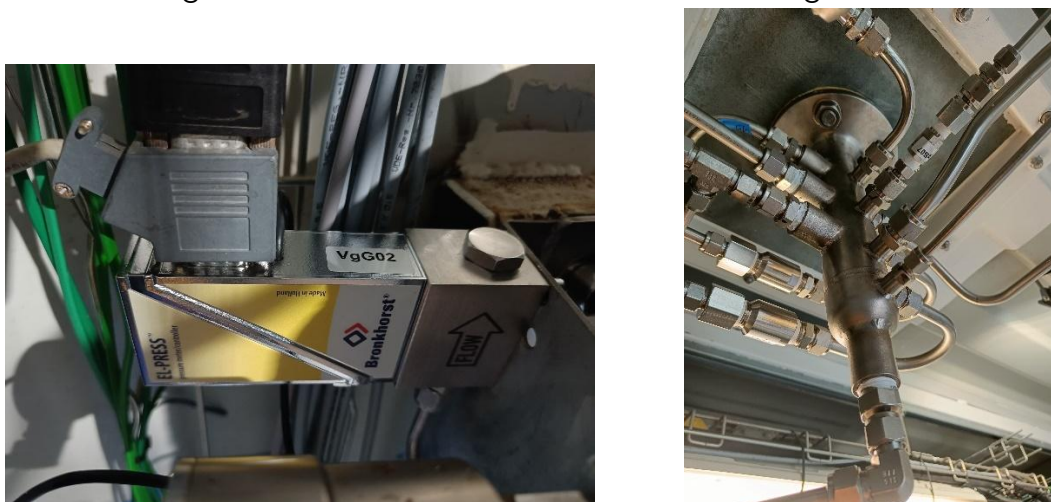
Figure 8: Example of new back pressure regulator and pressure relief valve used in StL-II
