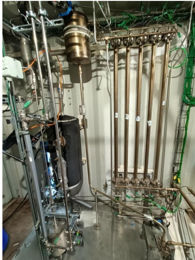
Figure 14: FT-reactor and separation section. Insulation has not been installed since the Notified Body (NoBo) must be able to do visual inspection of the pressure equipment.
